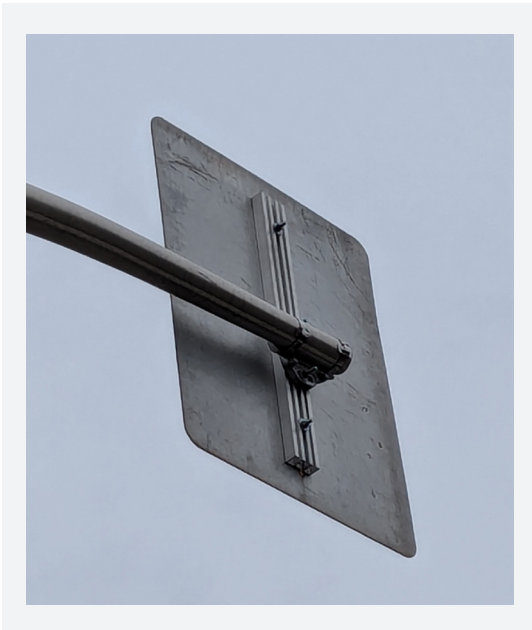
Mast arm bracket mounts road signs to overhead arms.
